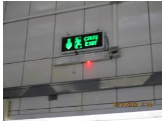
EMERGENCY EXIT SIGN.JPG
