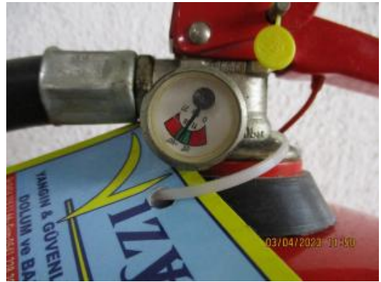
PRESSURE OF FIRE EXTINGUISHER.JPG
